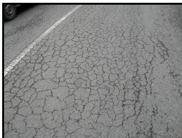
Alligator Crakes on existing Carriageway
