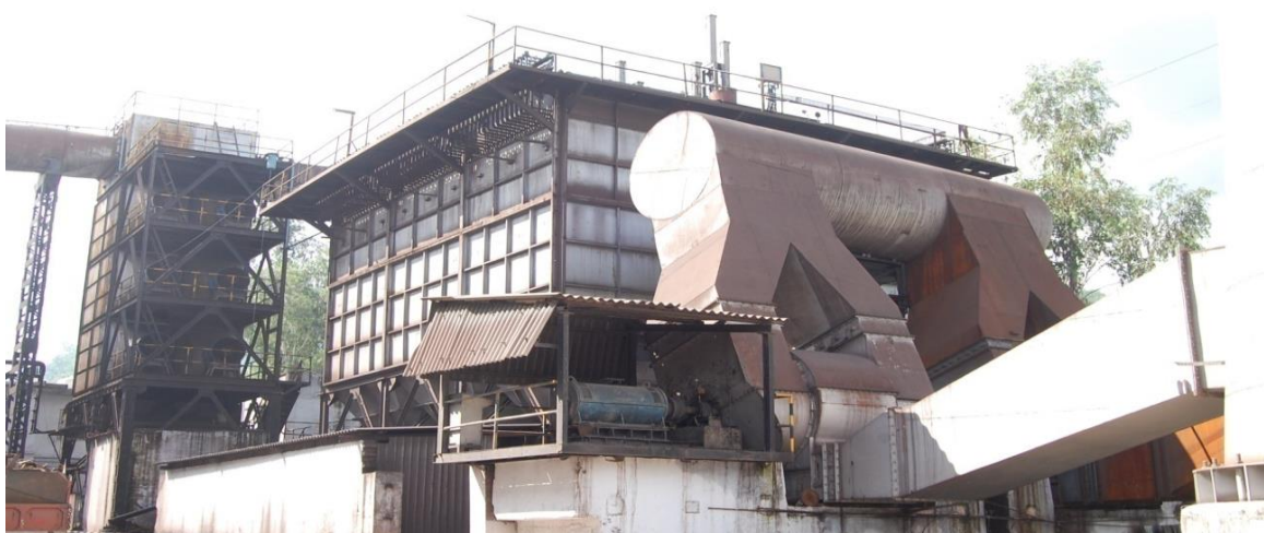
AIR POLLUTION CONTROL DEVICE
