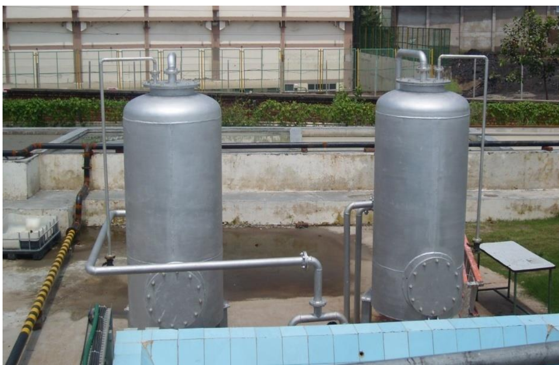
TERTIARY TREATMENT PLANT
