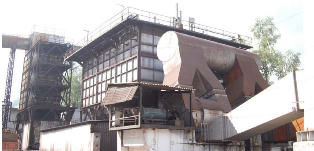
AIR POLLUTION CONTROL DEVICE
