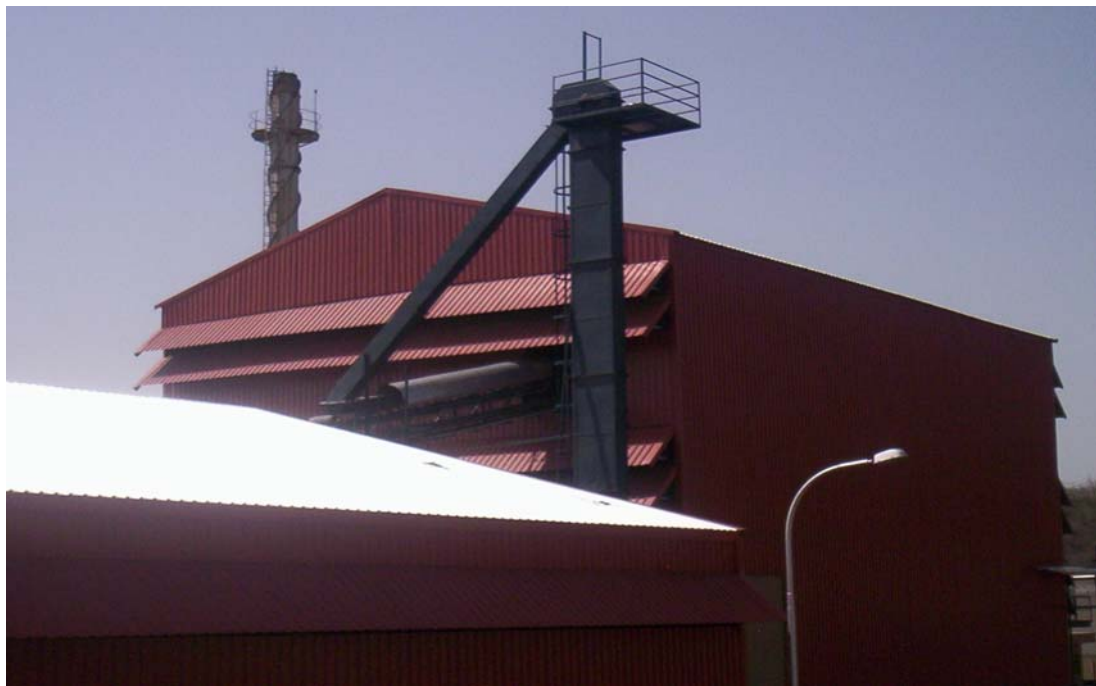
Figure – 4.8: Air pollution control system in boiler.
