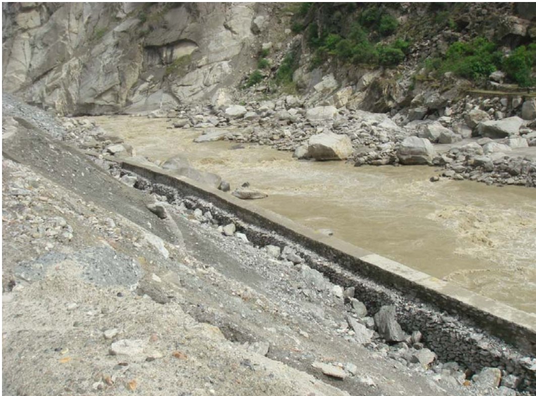
Figure – 4.1: Actual active dumping site with toe protection in a hydel project.
